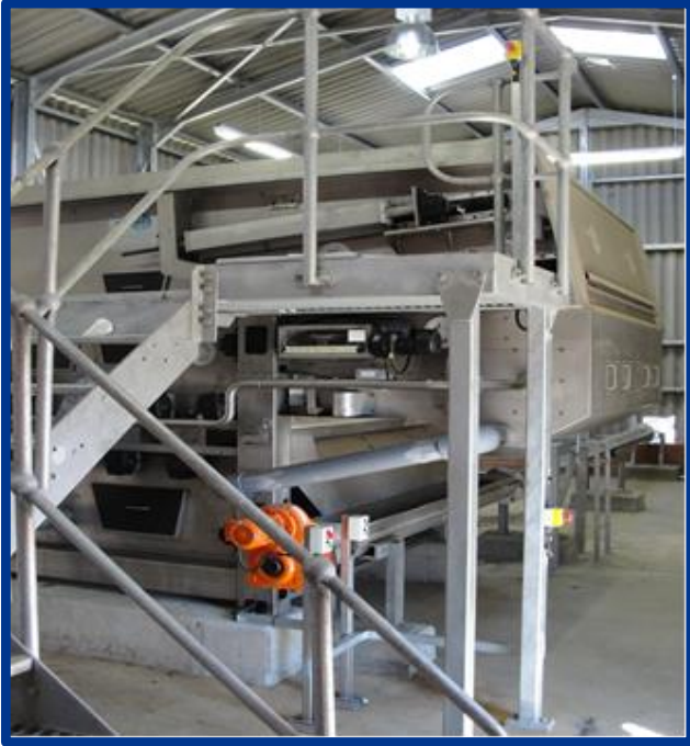
FILTER BELT PRESS AND ACCESS STRUCTURE
