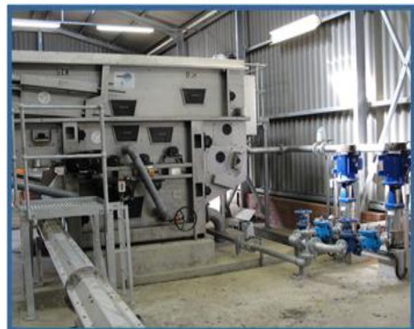
FILTER BELT PRESS AND SCREW CONVEYOR
