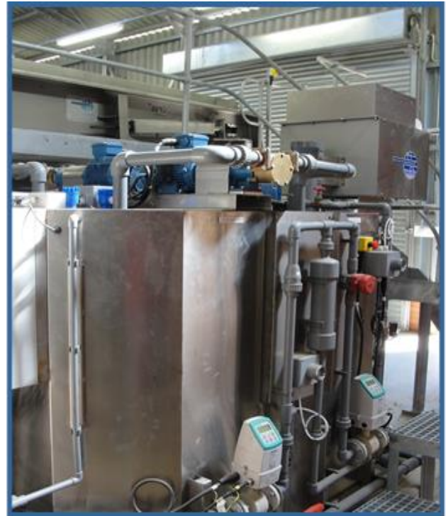
AUTOMATED POLYELECTROLYTE MAKE-UP AND DOSING PLANT
