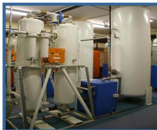
Receiver and Dryers
