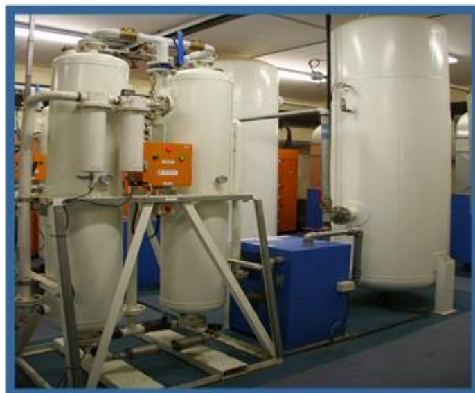
Receiver and Dryers
