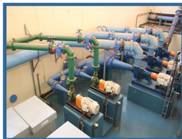
BACKWASH & RECIRCULATION PUMP STATION
