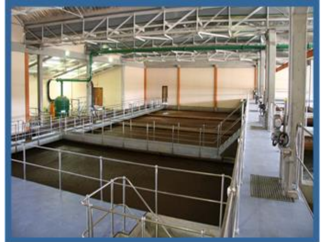
SATURATOR VESSEL & DAF TANKS
