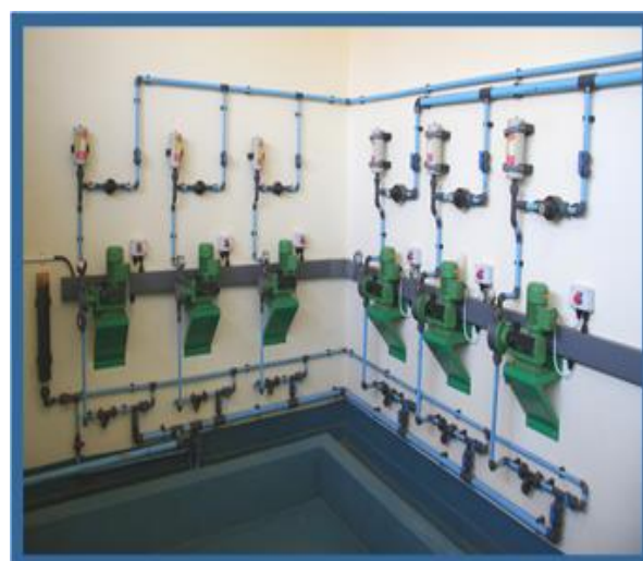
PRIMARY & SECONDARY FERRIC DOSING STATION
