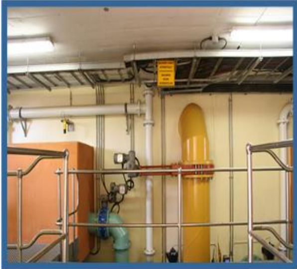
FILTER GALLERY PIPEWORK
