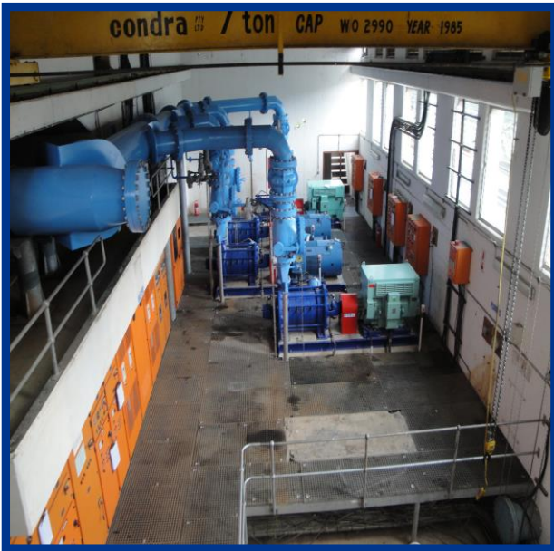
New pumps and manifold
