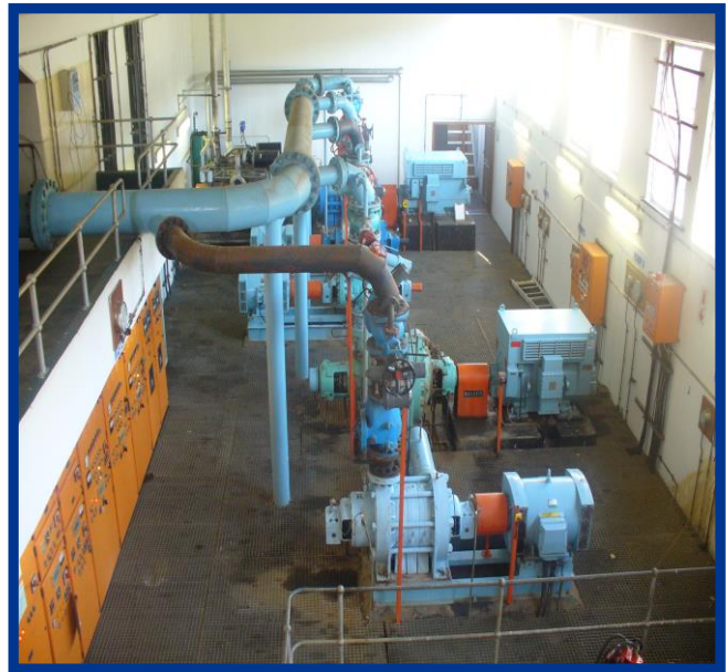
Old pumps and manifold
