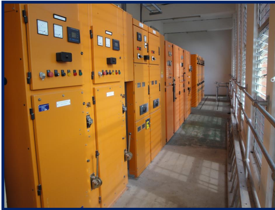
3.3kV panel, bus section and joggle chamber with new 22kV incomer and feeders in the distance
