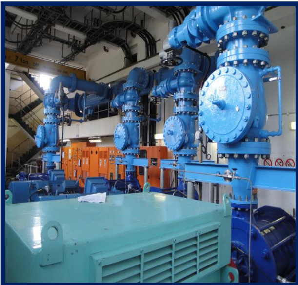
New 40 bar valves and pipework
