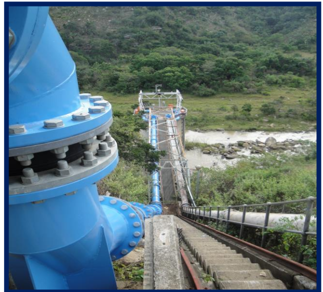
Low lift pipeline from high lift pump station down embankment and across bridge to caisson
