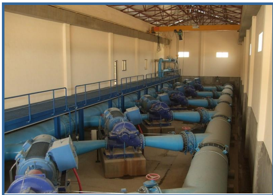
CLEAR WATER PUMP STATION
