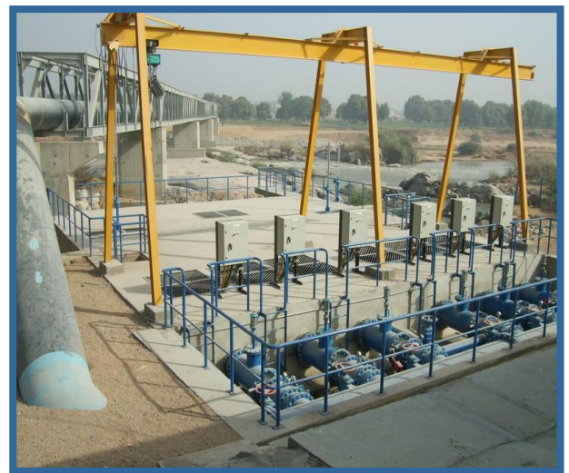
RAW WATER PUMP STATION
