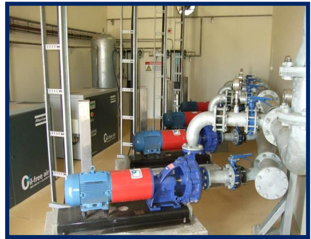
Cooling water pump station and additive air equipment
