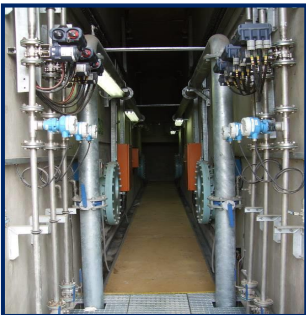
Main ozone contact tank gallery
