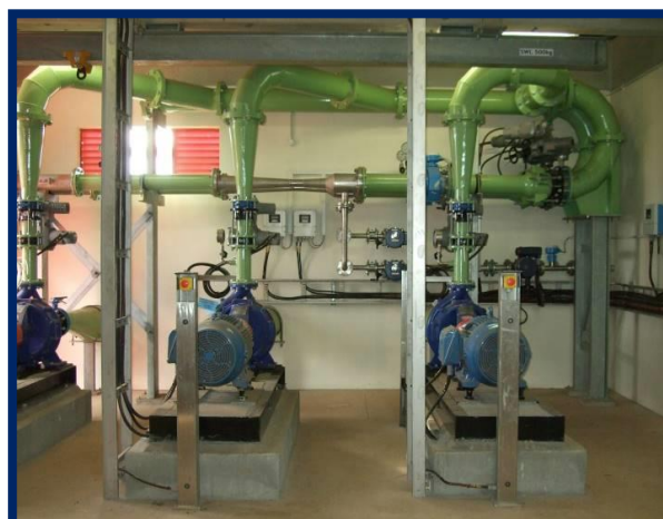
Pre-RGSF ozone side-stream injection pump station
