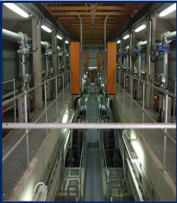
GAC filter building upper gallery
