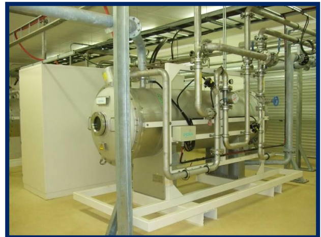
Ozone generator vessel and Power Supply Unit
