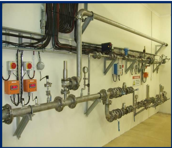
Ozone feed gas preparation
