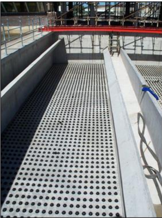
New monolithic rapid gravity filter under drains
