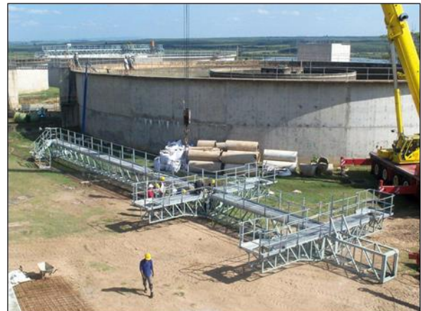
48m diameter clariflocculator bridge prior to installation
