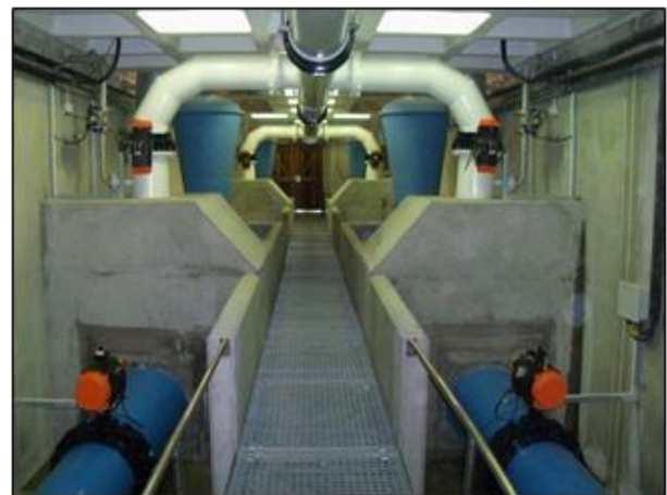
View of new filter gallery
