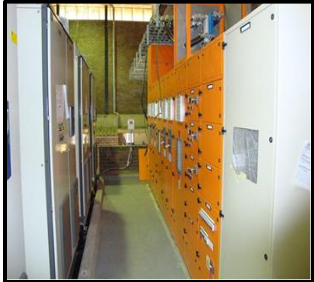
Electrical Motor Control Centres and Variable Speed Drives
