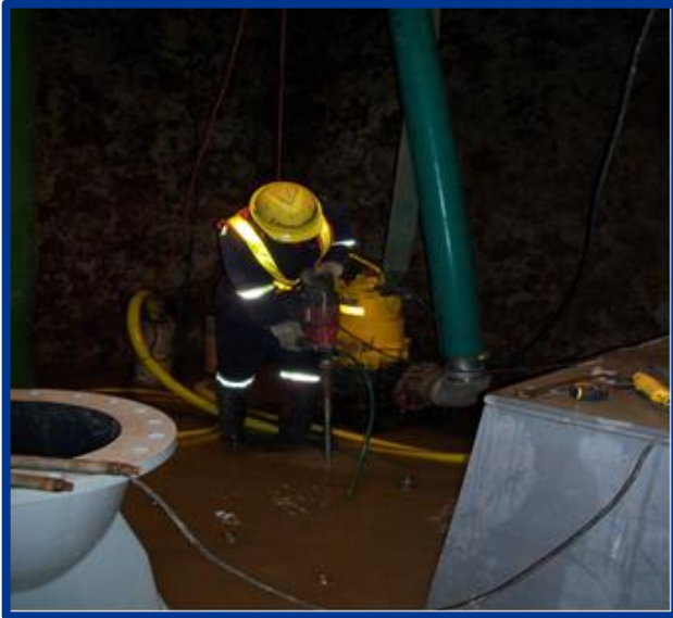
Preparing holding down anchors inside the Pump sump, with continuous dewatering required.
