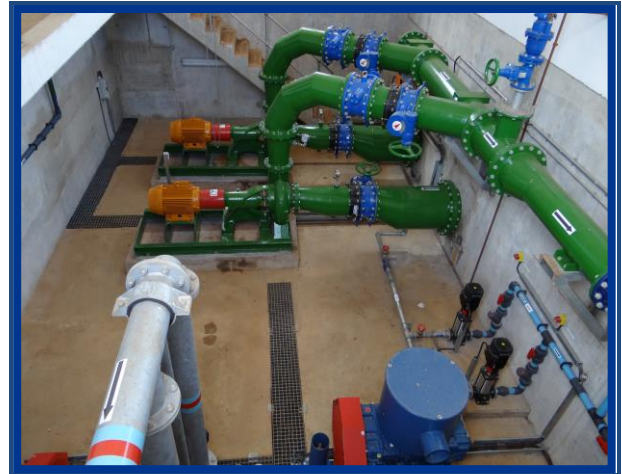
Backwash pump station
