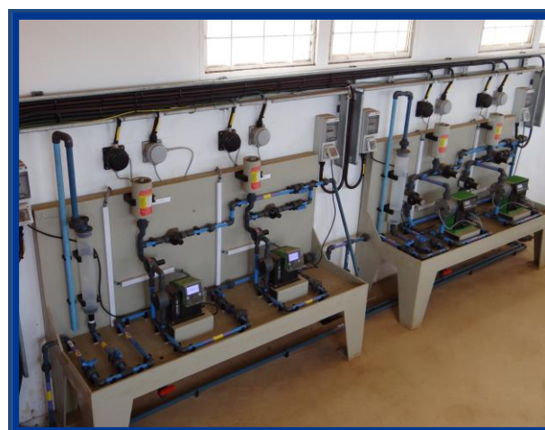
Chemical dosing equipment
