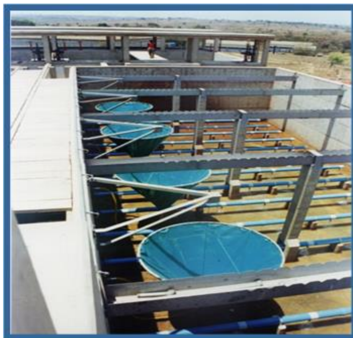
FLAT BOTTOM CLARIFIERS REFLECTING SLUDGE CONES
