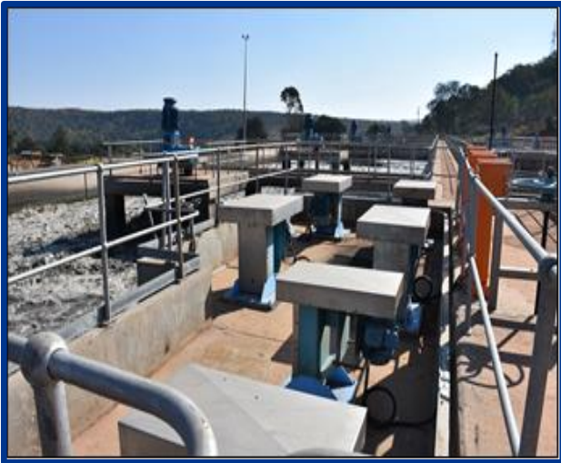
8 off vertical shaft mixers
