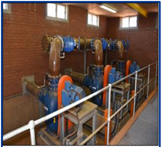
3 off Return Activated Sludge self-priming pumps
